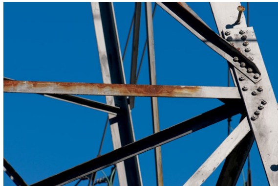
FIGURE 1.2: Rust that has degraded the surface of a structural element of a power transmission tower [18].
