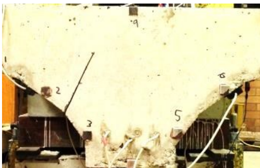
Figure 4. Damage case 2, (150 × 50) mm cut in the concrete
