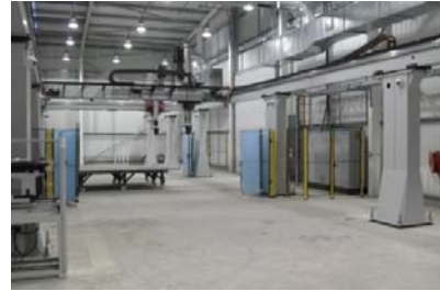
Figure 2 - Photo of FreeFAB Wax gantry installed at GRC UK plant, UK (courtesy of Laing O'Rourke)
