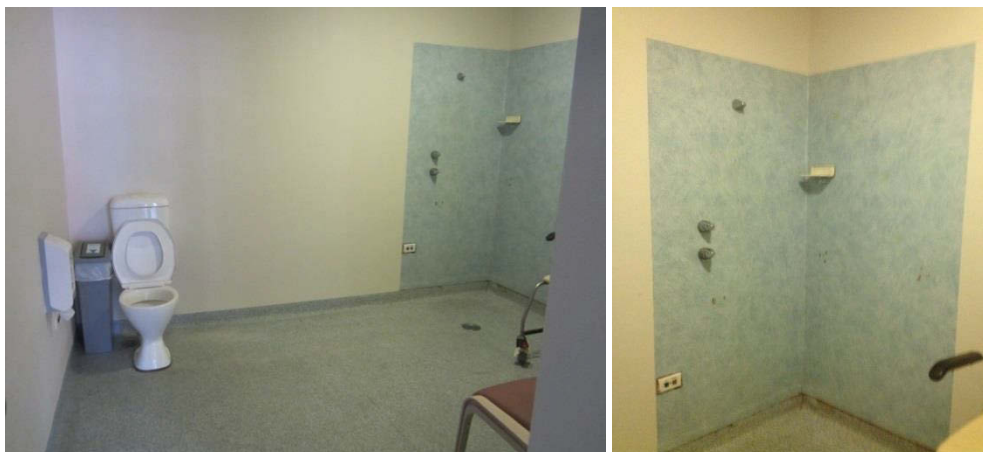
Image 7.10: Worn, hazard controlled bathrooms/shower detail
