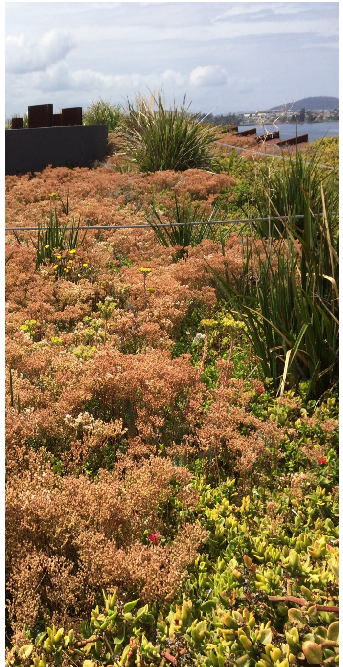
Green roof, MONA, Hobart (source: P. Osmond, n.d.)
