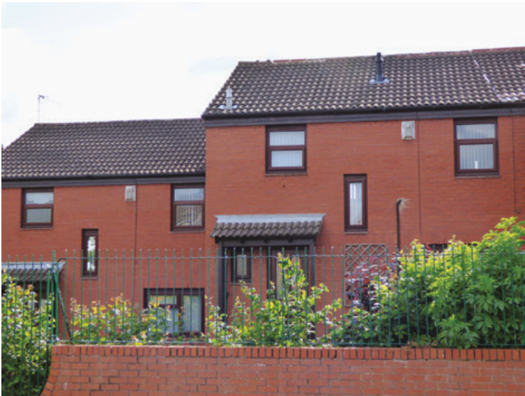
Figure 12.2 Weller Street Co-op resident-led design, well managed and in better condition today compared with surrounding housing built afterwards.
