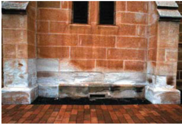
Figure 2.4. Salt and water damage resulted from a sandstone building (Department of Environment and Climate Change NSW 2008a)
