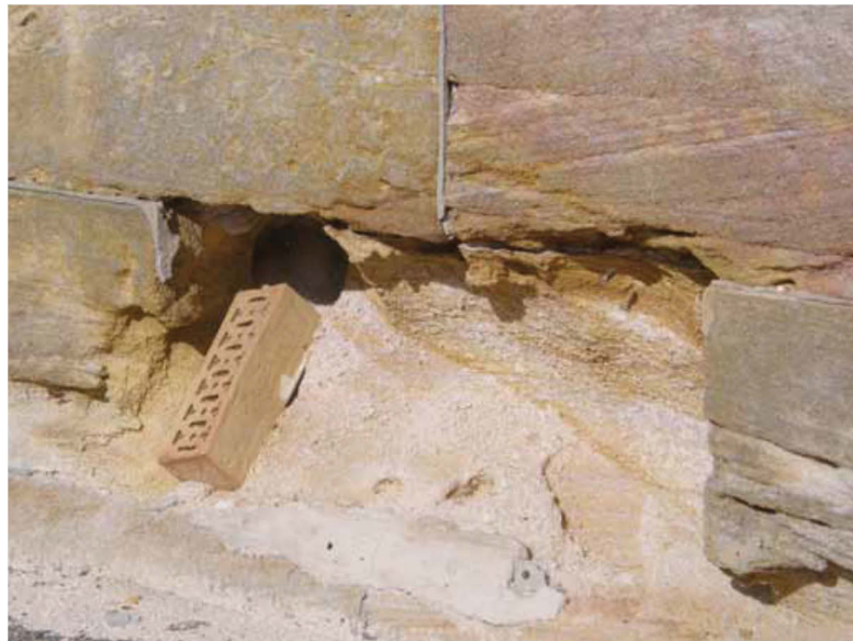
Figure 2.2. Image showing salt attack as found from disaggregated sandstones buildings on Sydney Harbour's Spectacle Island (Swann 2011)
