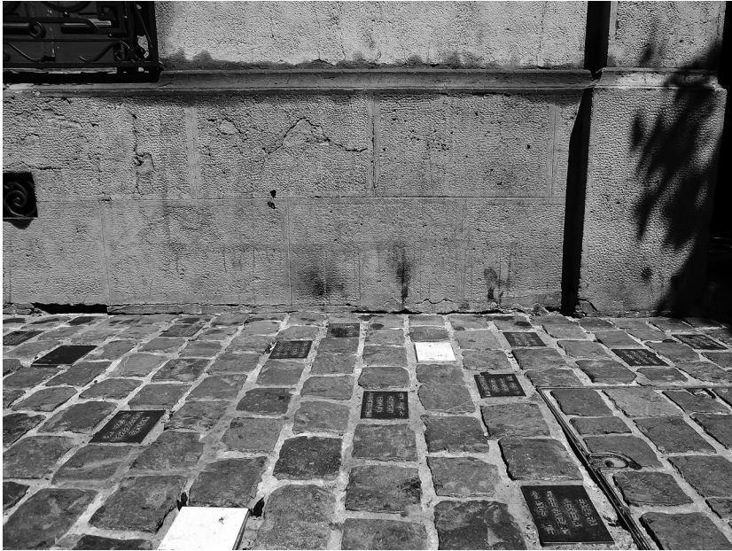
The front façade, Londres 38, showing the marks of burning candles resting against it during the vigils held for the detained-disappeared.
