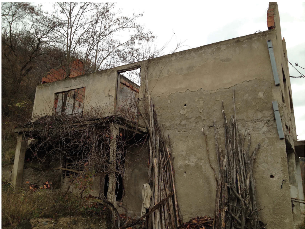
Figure 135: Demolished house in Banjska (Nevena Mrdjenovic 2013)
