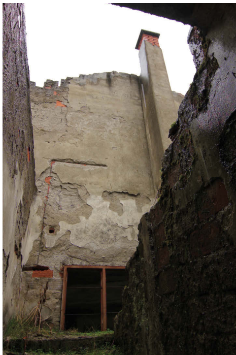
Figure 115: Roofless house near Derventa (Nevena Mrdjenovic 2013)
