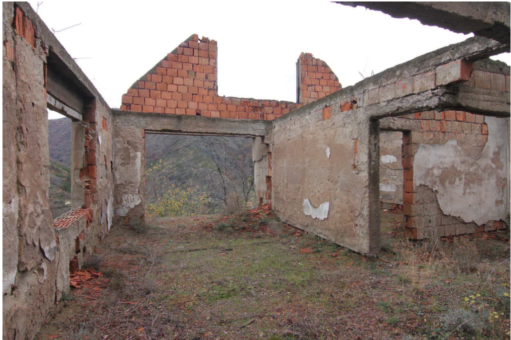
Figure 134: Destroyed house in Banjska (Nevena Mrdjenovic 2013)
