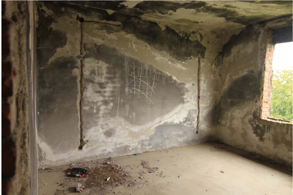
Figure 108: Vandalised walls in a former bedroom (Nevena Mrdjenovic 2013)
