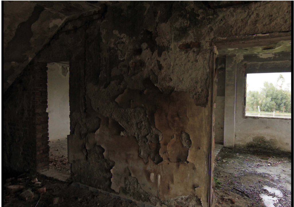
Figure 105: Abandoned and stripped houses (Nevena Mrdjenovic 2013)
