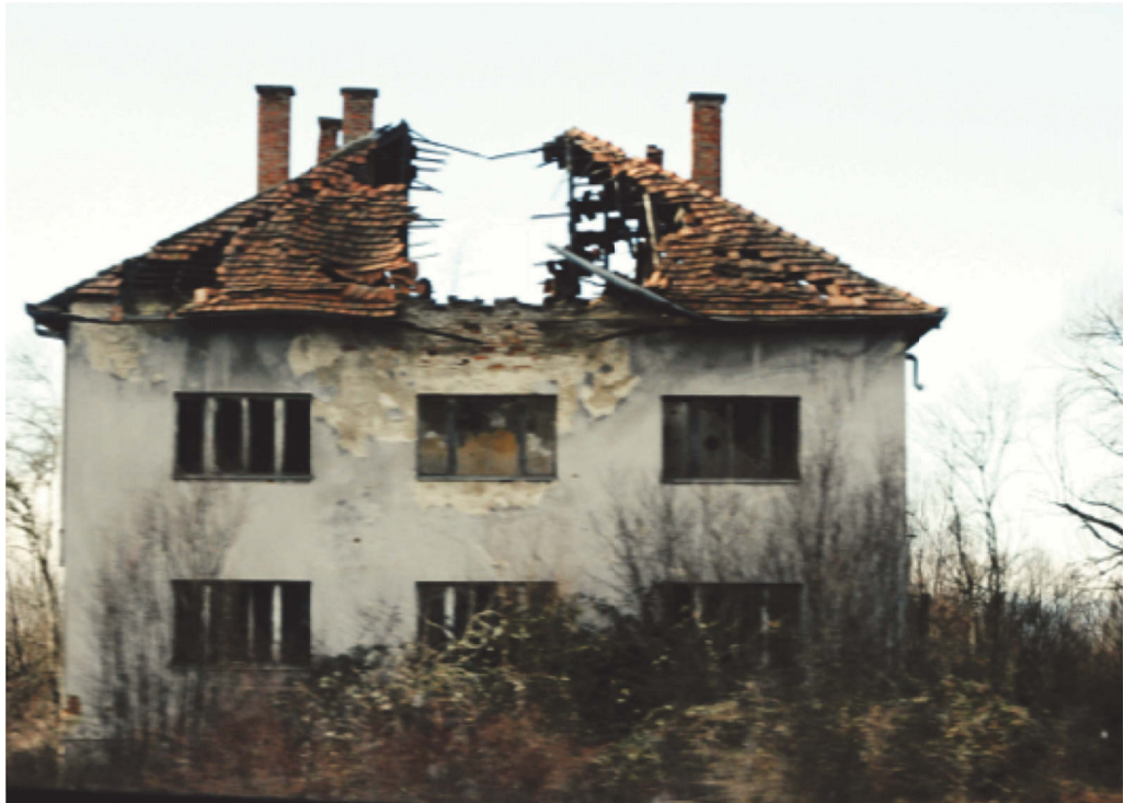
Figure 96: Smashed house on E-661 (Nevena Mrdjenovic 2012)
