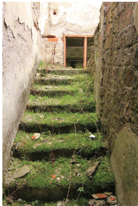
Figure 116: Staircase in a roofless house (Nevena Mrdjenovic 2013)
