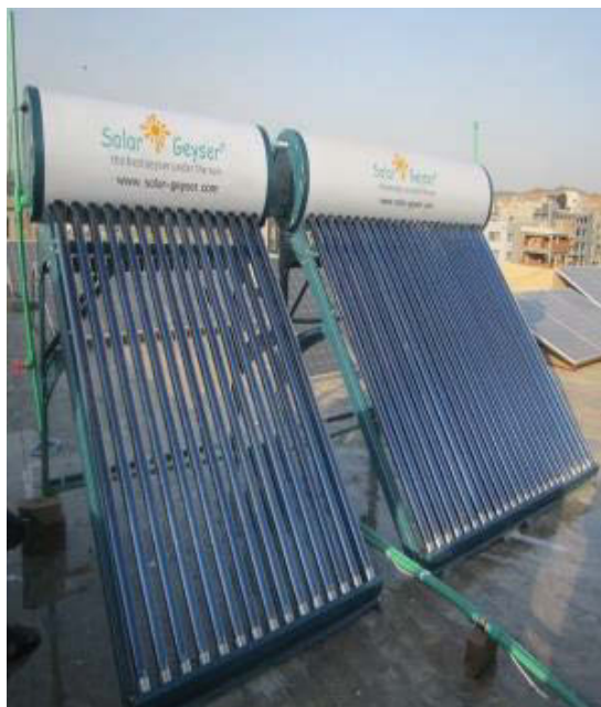
Figure:1.14: An example of Water Heating based on Solar Energy – Domestic Solar Water Heater (Source: Photo taken from www.solar-geyser.com )
