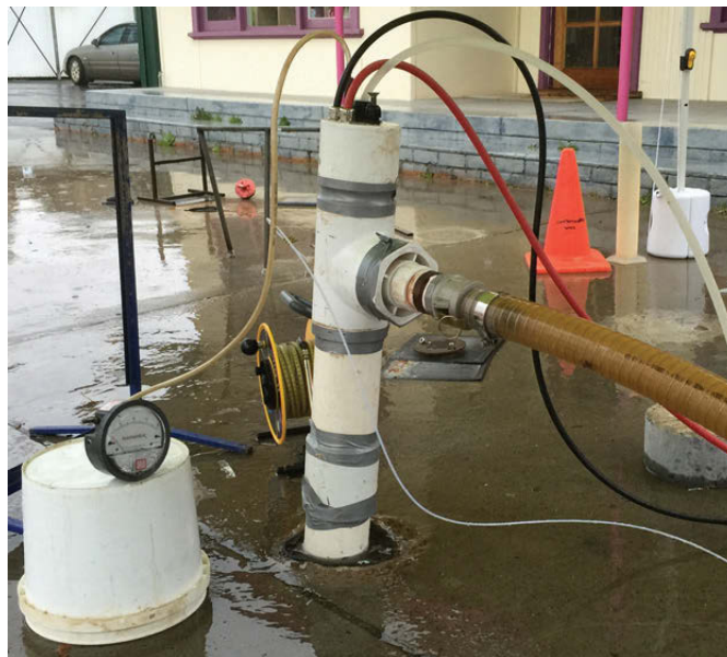
Figure 3. 15. Arrangement of well head for water and vacuum enhanced recovery at well PB40.
