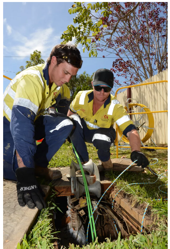
Workers layout cable as part of the NBN roll-out, which has caused controversy with recent revelations of asbestos mismanagement. AAP
