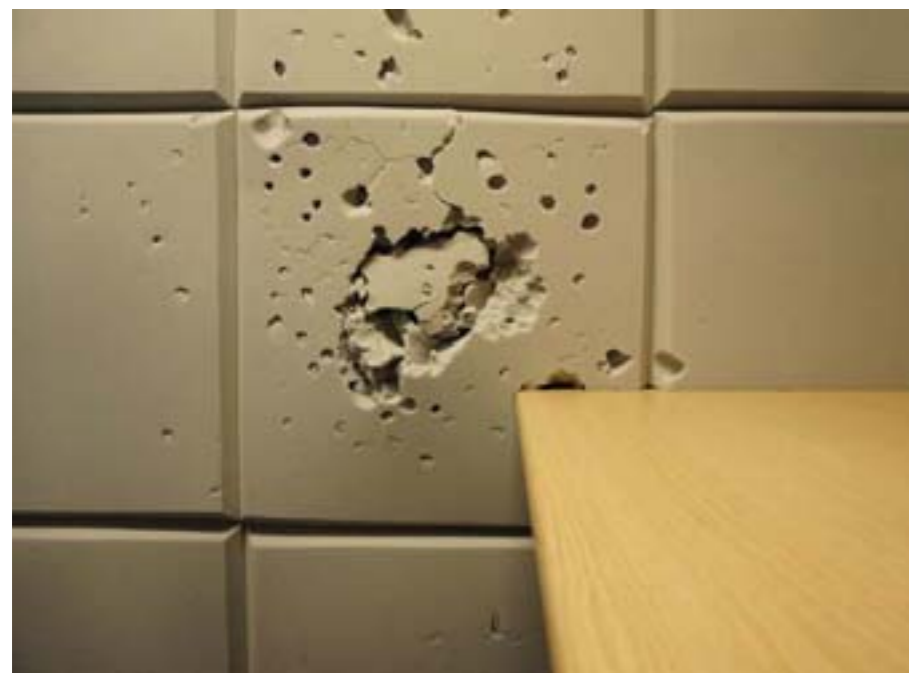
Torn soundproofing in a Cobham AVL studio
