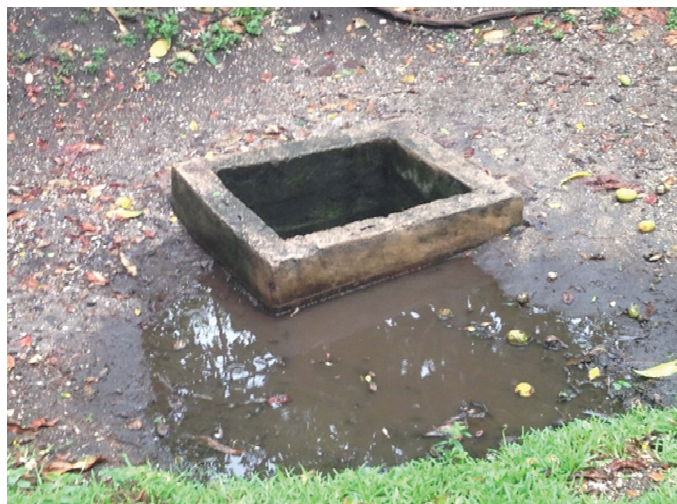
Figure 13. Pooling around well in Uripiv
