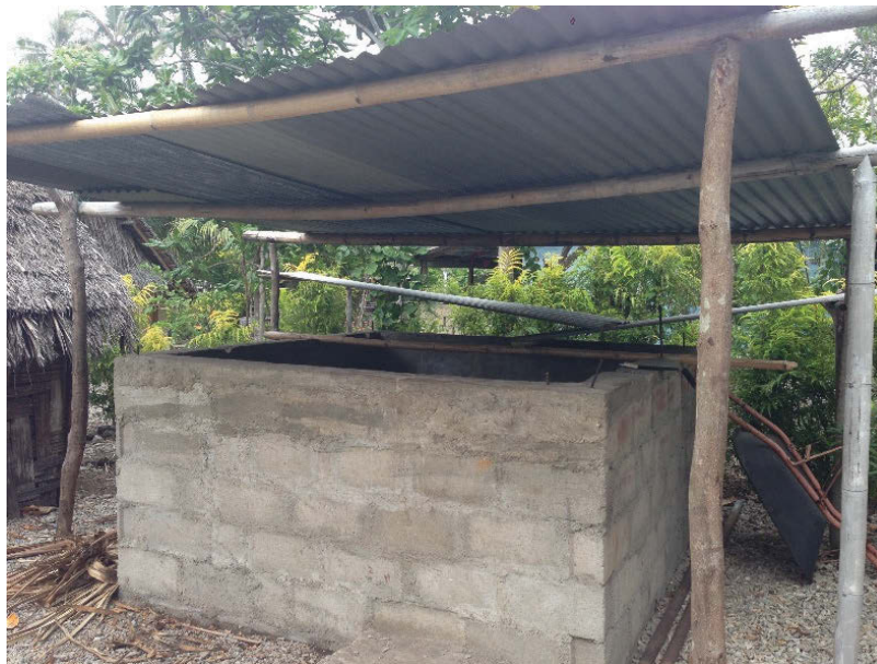
Figure 14. Underground rainwater storage tank (lasitern) in Uripiv
