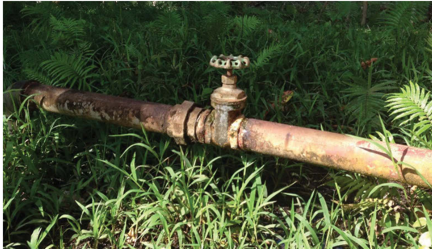
Figure 12. Namoru community water main
