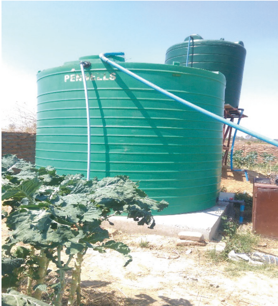
Figure 11: Part of the irrigation infrastructure ( Photographs taken by researcher 2016 )
