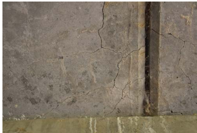
Figure 1. Cracking of bridge beams due to ASR
