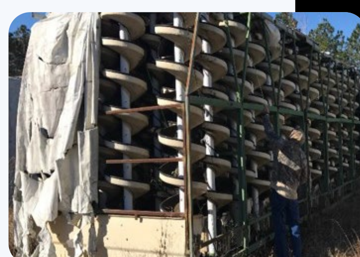
Bank of GSS operating in the field
