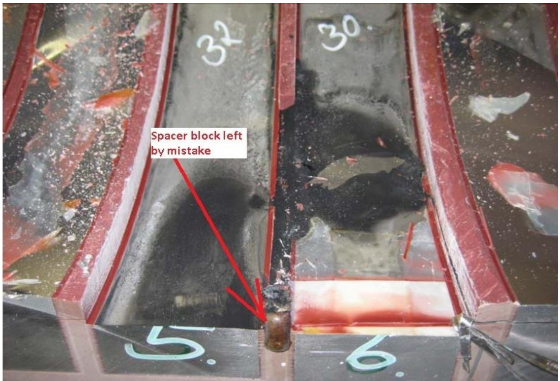
Figure 4-14: Damages in both single 33 kV windings beside the foreign material (courtesy of Aurecon).
