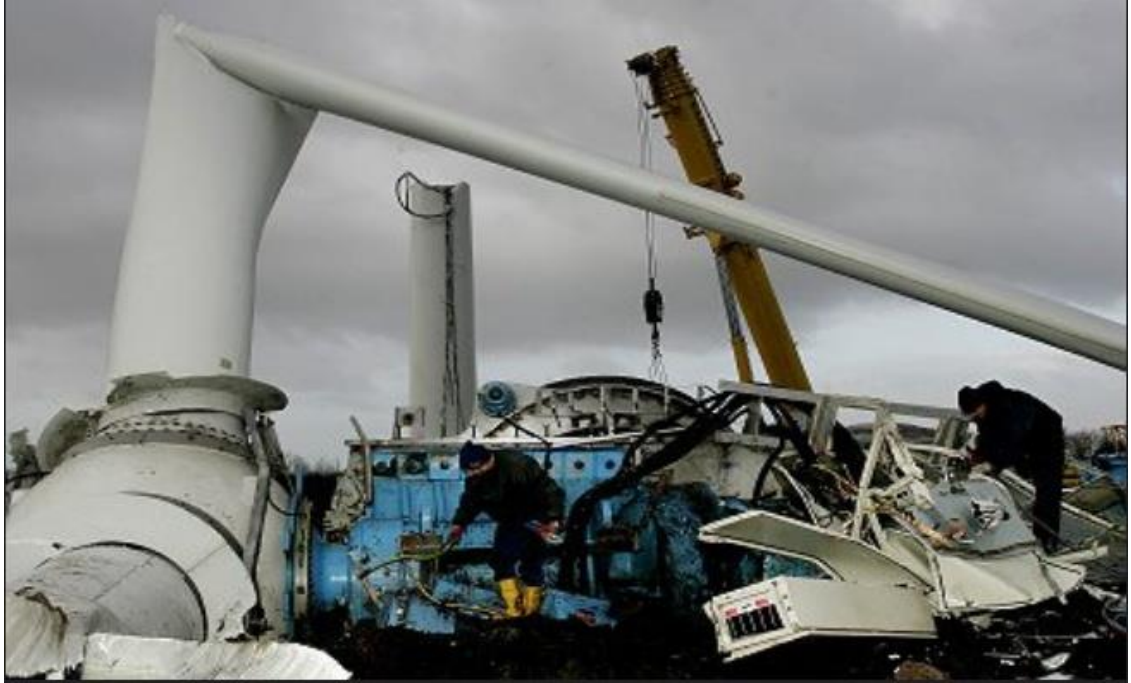
Figure 4-7: Wind turbine mast failure (Photo: https://www.flickr.com/photos ),
