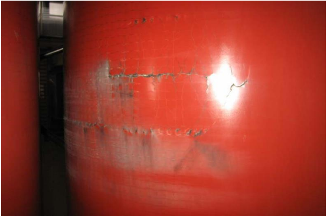
Figure 4-13: 690 V / 33 kV transformer failed HV coil (courtesy of Aurecon).
