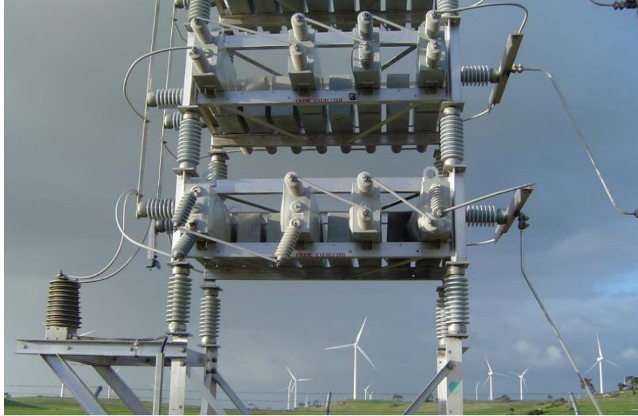
Figure 4-19: Capacitor bank failure (courtesy of Aurecon).
