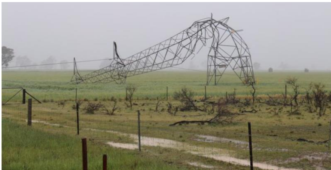
Figure 2-63: Collapsed electricity tower in South Australia (Photo: ABC News, Tom Fedorowytch 29/09/2016).
