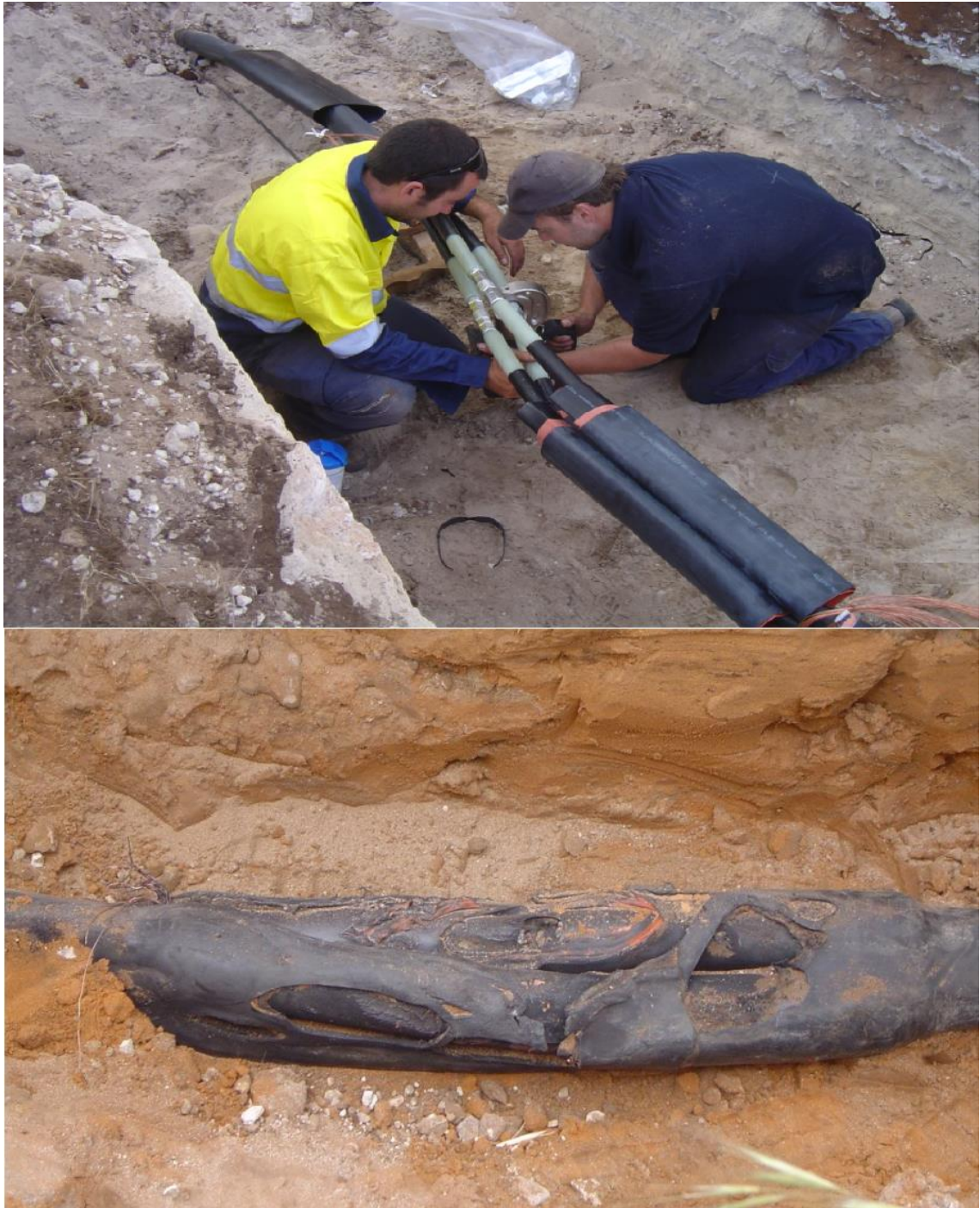
Figure 4-16: Three core 33kV cable joint failure (before and after) (courtesy of Aurecon).
