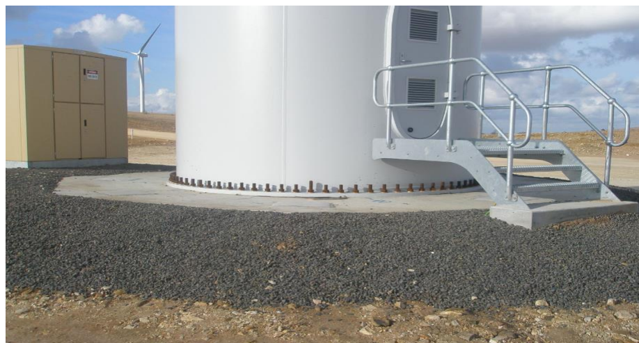
Figure 3-41: Wind turbine base (courtesy of Aurecon).
