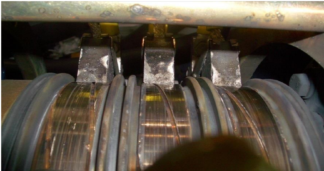
Figure 4-10: Slip ring and brushes after failure event (courtesy of Aurecon).
