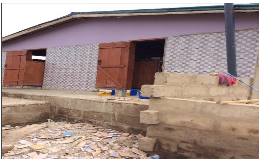
Plate 7.6: Adapting Community Toilet due to Flooding by raising Foundation in Old Fadama
