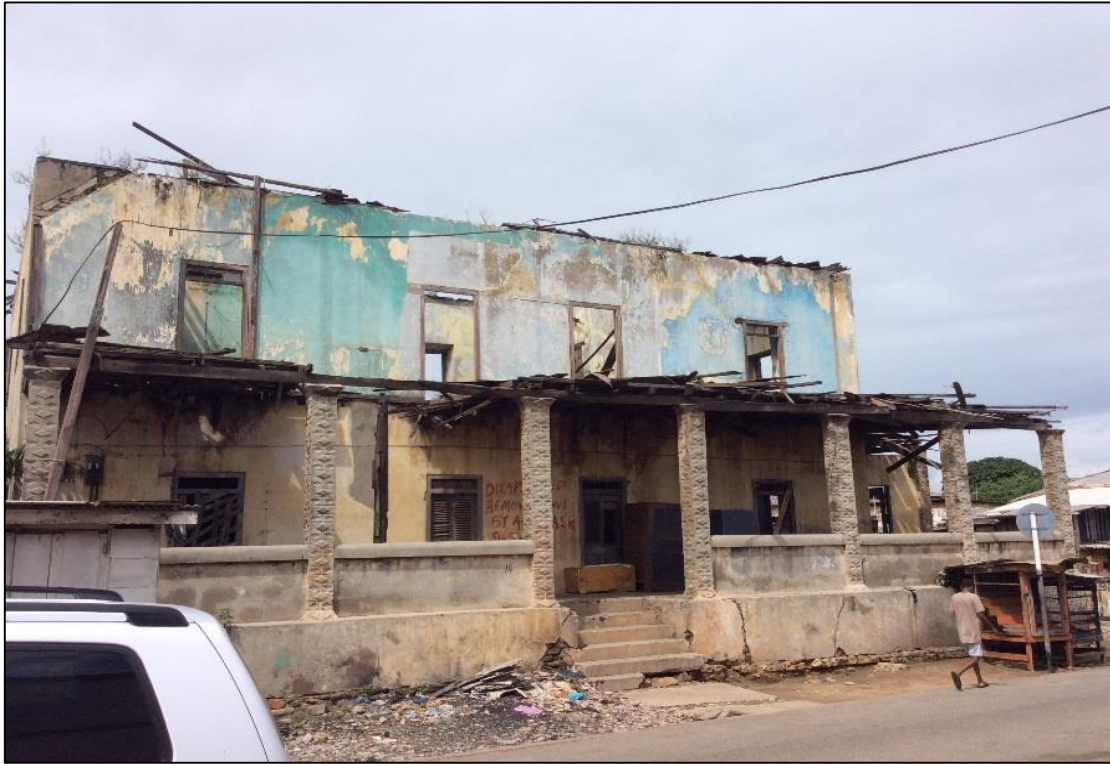
Plate 5.4: Ripped off Roofs in Adedenkpo
