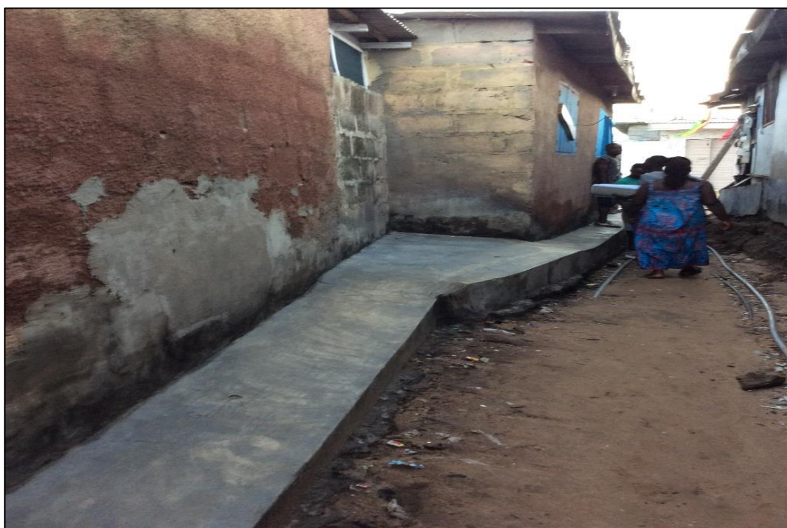
Plate 7.5: Responding to Flood by protecting Foundation with a curb in Gbegbeyise
