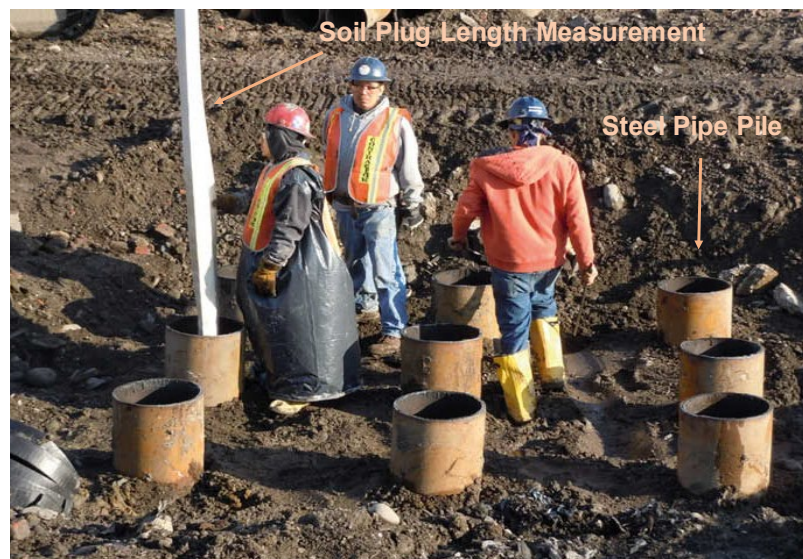
Figure 2.3 Driven steel pipe piles and the measurement of soil plug length (after Fattah & Al-Soudani 2016)
