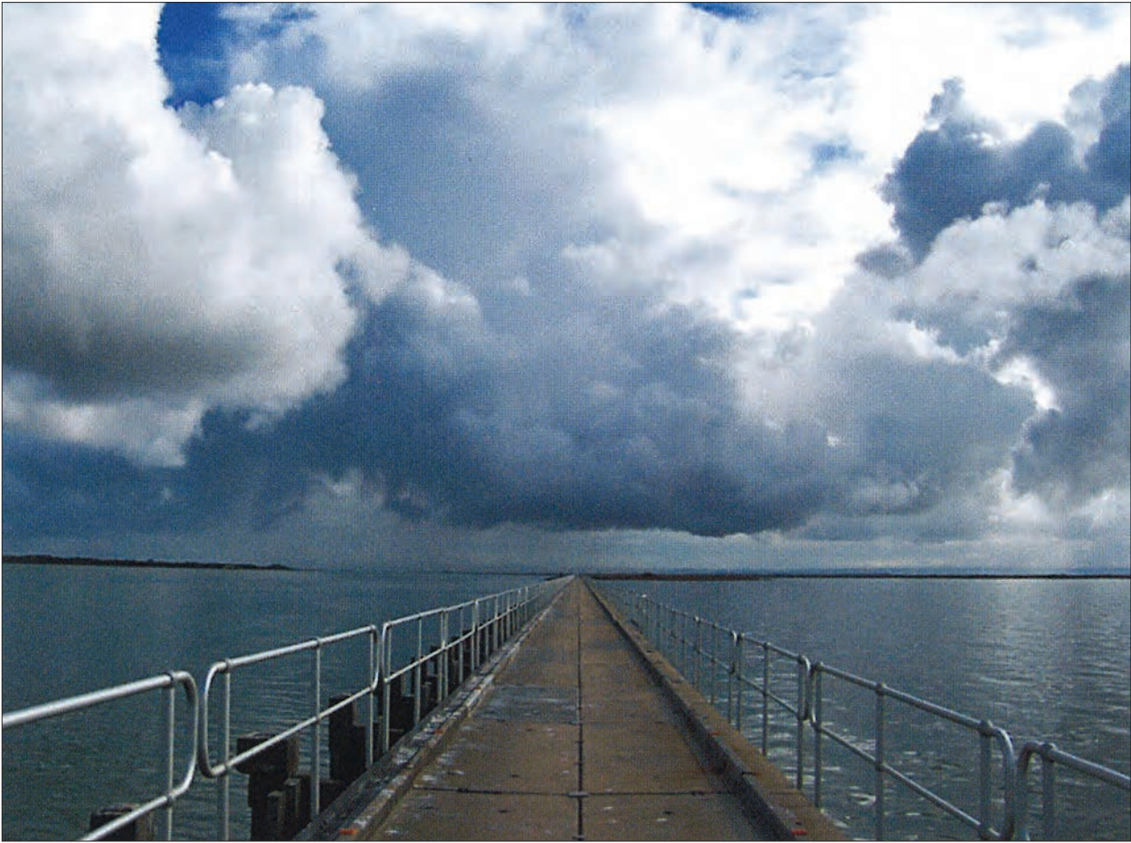
Figure 1.1.15 Tauwitchere Barrage near the Murray River mouth. (From Ngarrindjeri Nation (2007), courtesy of David Sjoberg)
