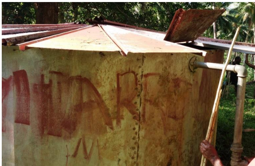
Figure 11. Namoru community water storage tank
