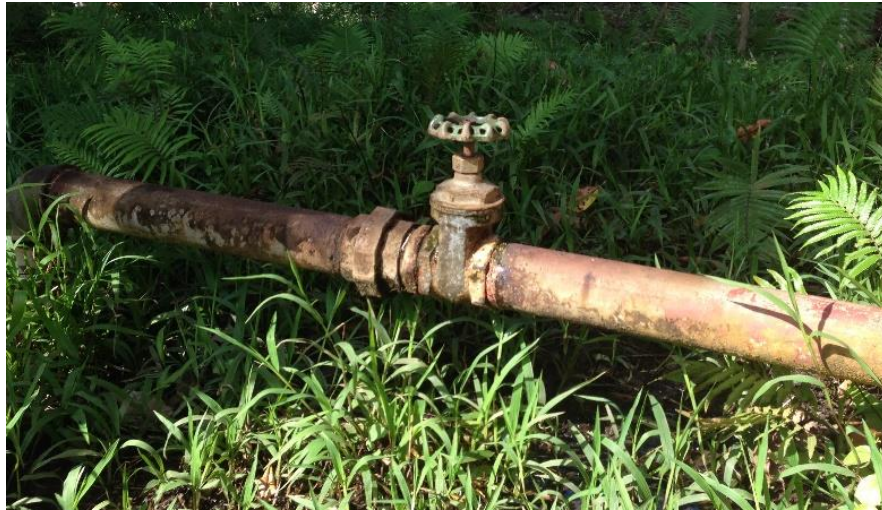
Figure 12. Namoru community water main
