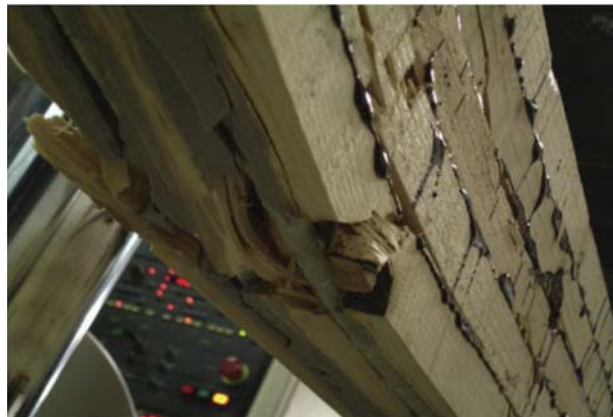
Figure 2-14 Tensile fracture by defect in bottom lamination (Raftery and Whelan 2014).
