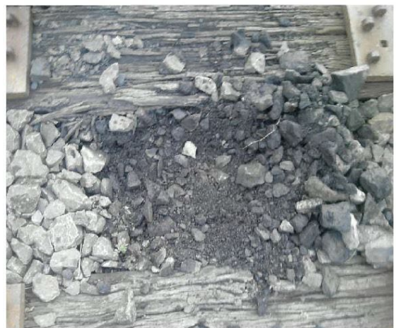
(ii) Enlarged view showing ballast breakage
