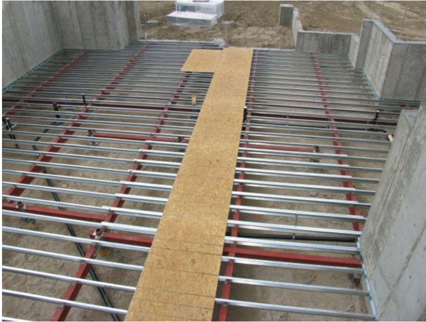
Figure 1 : Typical set out of a cold-formed steel and timber composite flooring system
