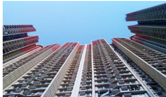
Split-system air conditioning units on the façade of a residential high-rise in Kowloon, Hong Kong. Source: https://www.tugraz.at/en/tu-graz/services/news-stories/tu-graz-news/singleview/article/architektonische-loesungen-statt-klimaanlagen/
