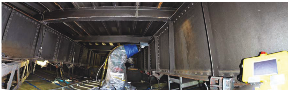
Figure 2.14: A robot set up and ready to blast a section of the Sydney Harbour Bridge.
