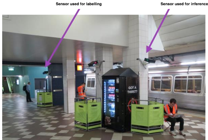
Figure 4: Sensors mounted at train station
