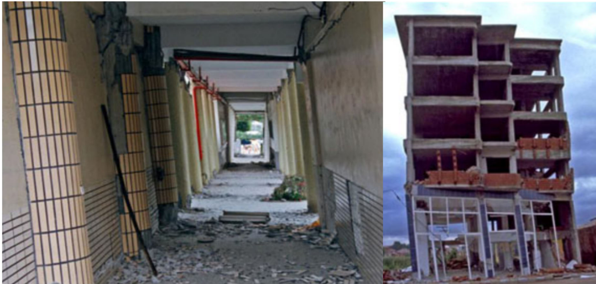
Figure 2.22 Examples of buildings with considerable residual displacements, leading to demolition (Ramirez and Miranda, 2012)
