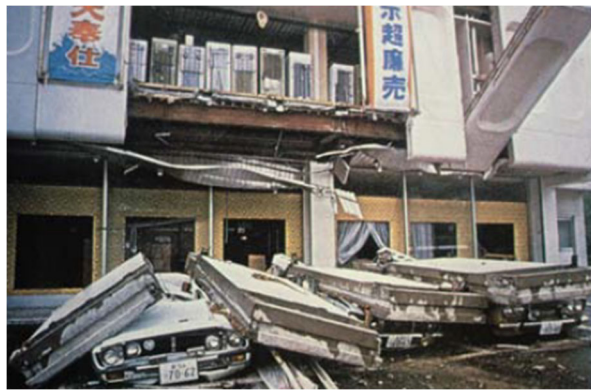
Figure 2.21 Fallen concrete curtain wall panels in 1978 Miyagi earthquake (Ishiyama, 2011)
