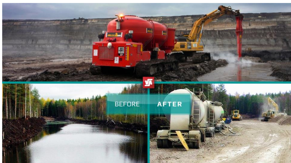
Figure 1.1: Requirements for construction in inappropriate ground profiles (Soil Stabilisation System, viewed 22 November 2019, < https://allustabilization.wordpress.com/ >)
