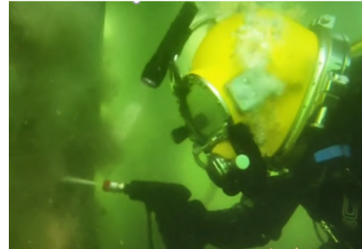
Fig. 1: Diver on cleaning operations
