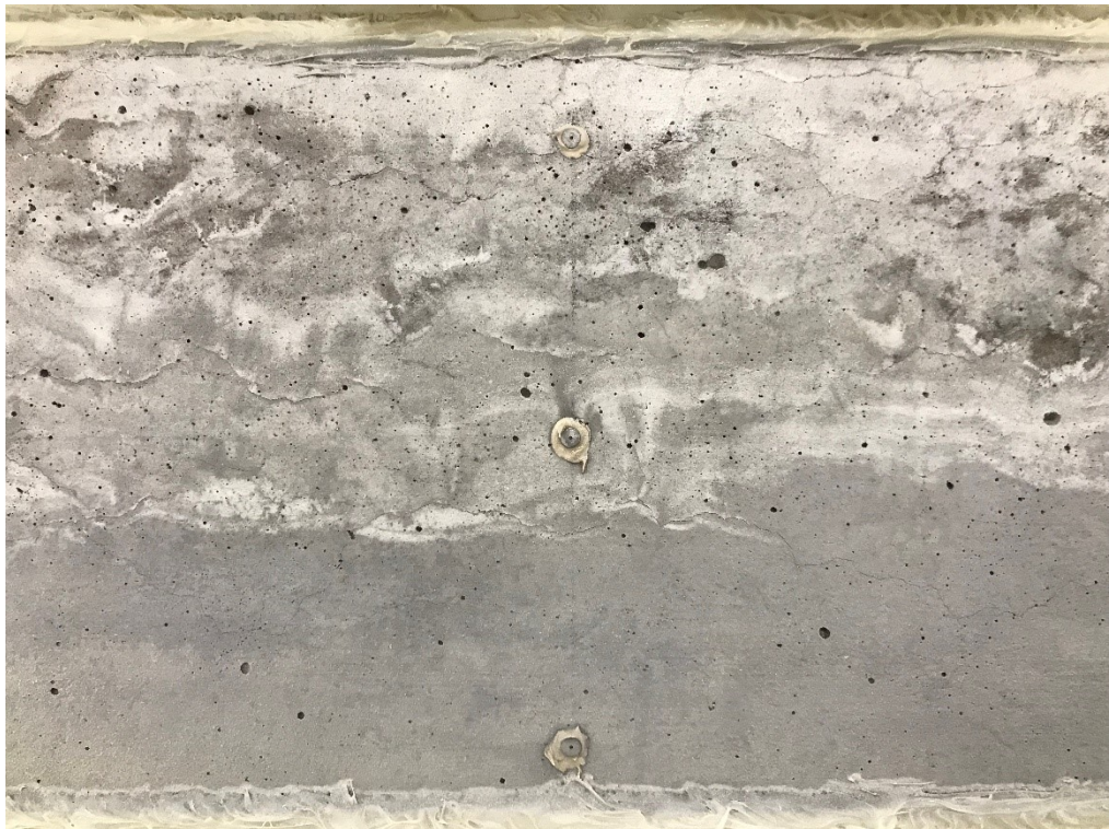
Figure 7. 30 Cracking on R1 beam surface (photo taken on 31/03/2020, 12 th month)
