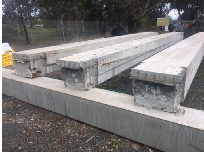
Figure 3. 2 ASR affected bridge beams from a demolished bridge deck
