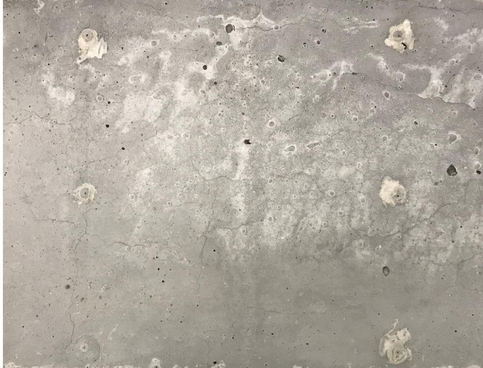
Figure 7. 29 Map cracking on R1 beam surface (photo taken on 31/03/2020, 12 th month)
