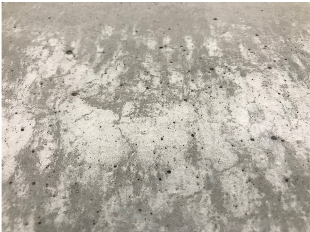
Figure 7. 28 Cracking on R1 beam surface (photo taken on 30/09/2019, 6 th month)
