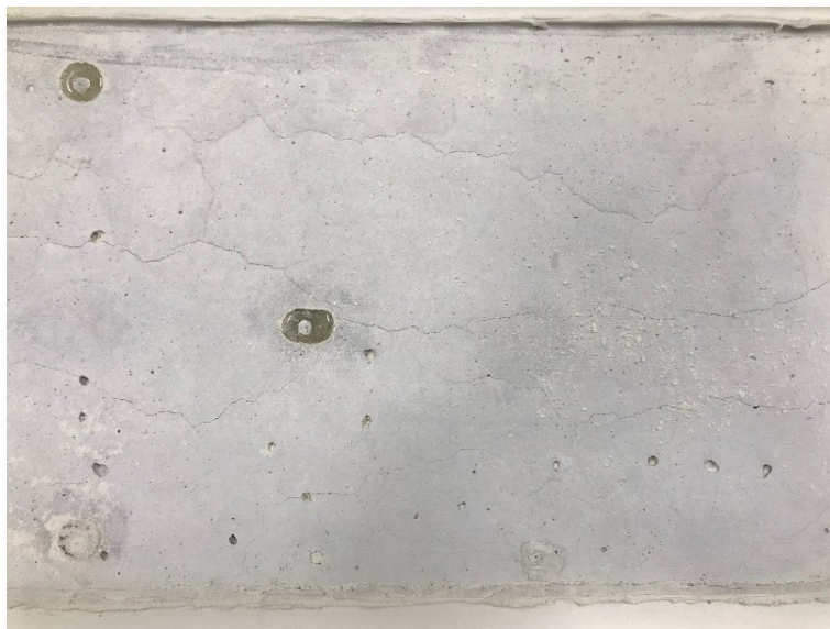
Figure 7. 33 Longitudinal cracking on R2 beam surface (photos taken on 31/03/2020, 12 th month)
