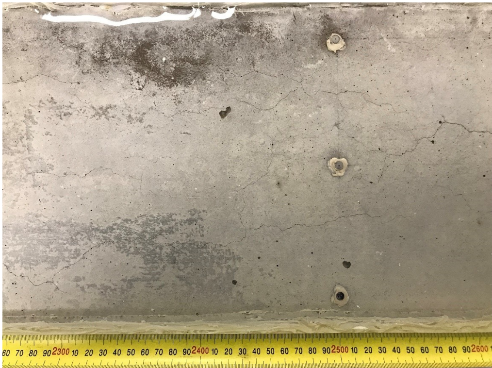
Figure 7. 32 Cracking on R1 beam surface (photo taken on 10/08/2020, 500 days)
