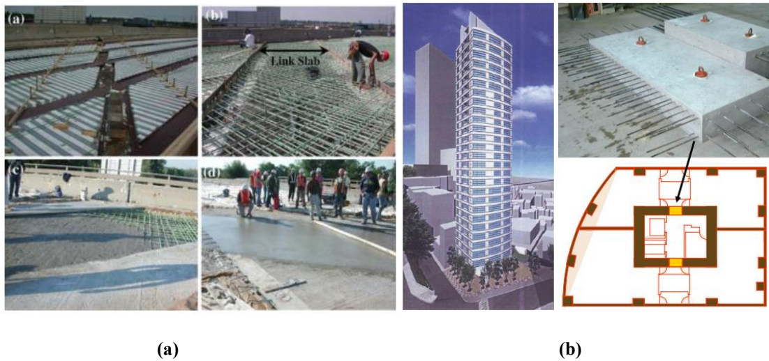
Figure 1.8 Application of SC-ECC: (a) Link slabs of bridge deck in Michigan, USA (Lepech & Li 2009); (b) Coupling beams in the core region of multi-storey structures in Japan (Maruta et al. 2005).
