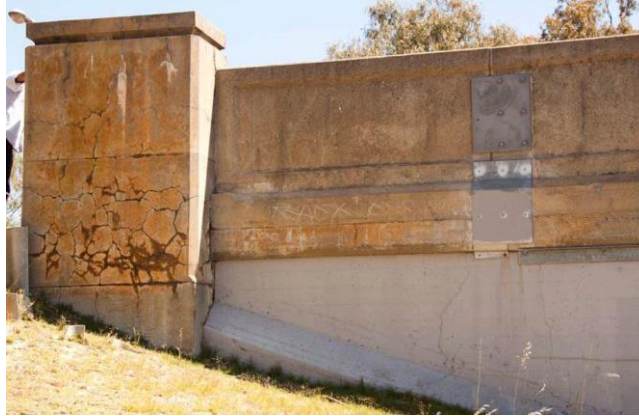
Figure 1.2: Causeway bridge affected by ASR in Perth, WA (HB79 2015)
