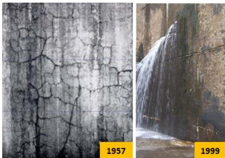
Figure 2.11 The Chickamauga lock and dam showing extensive cracking due to ASR (dominating mechanism) and ACR (Smith et al. 2017)
