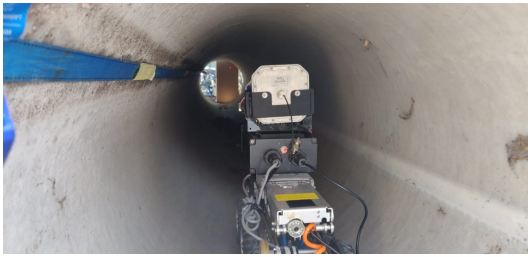
Fig. 3. Robot traversing inside the pipe for collecting UHF-RFID sensor wireless signals.
