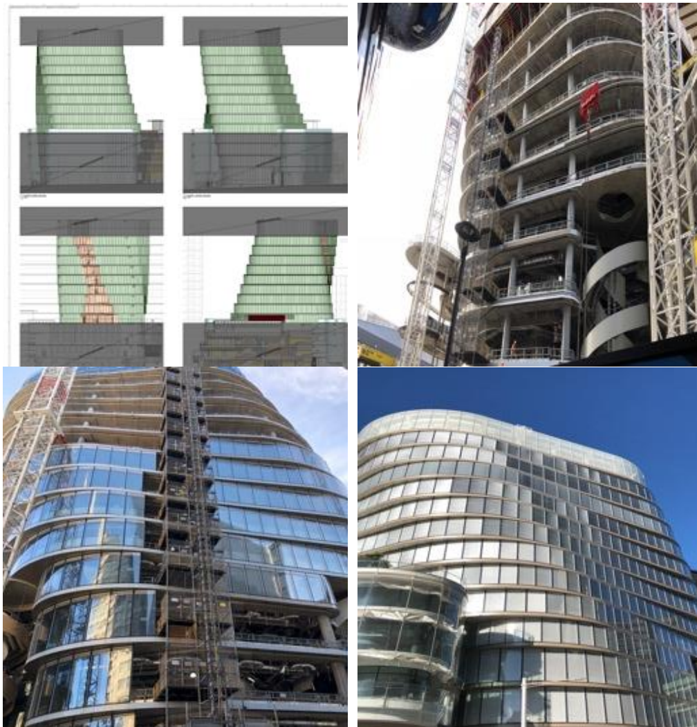
Figure 6-1 Case study A – Photos of the CCF façade at different construction stages
