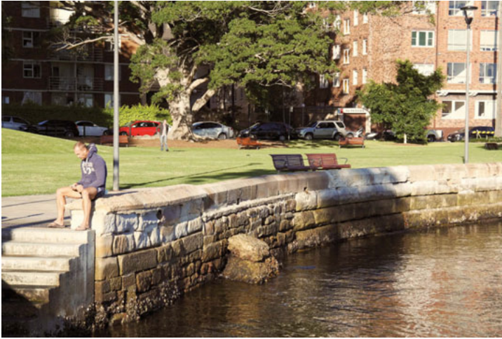
Figure 2. The Elizabeth Bay sea wall and reclamation from the east. (Denis Byrne 2015)
