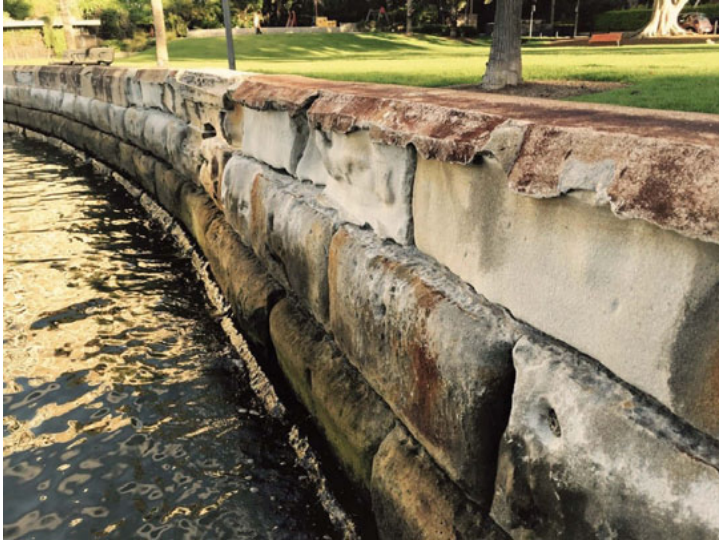
Figure 4. A section of the seawall showing severe erosion of some of the sandstone blocks. The top of the wall in the foreground was capped with concrete mortar several decades ago, subsequent to which the sandstone tier directly below has continued to erode landwards (Denis Byrne 2016)
