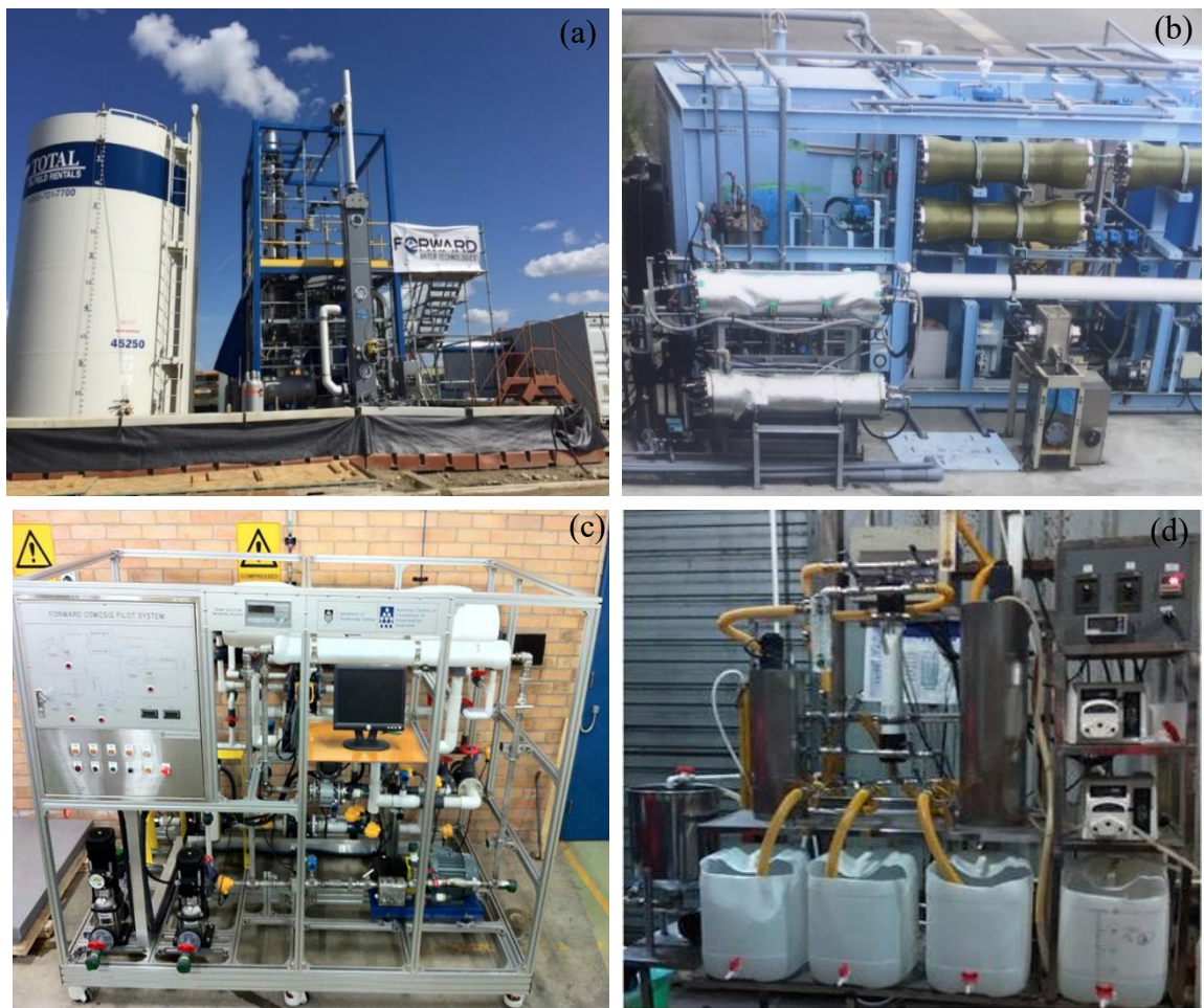
Figure 2.8: Pictures of (a) A full-scale FO plant in Airdrie, Alberta (Canada) [181] (b) A pilot FO plant at Nagasaki (Japan) (c) A pilot FO plant at University of Technology Sydney [110]; and (d) A pilot FO plant at the Quyang Municipal Wastewater Treatment Plant (WWTP), Shanghai (China) [182].
