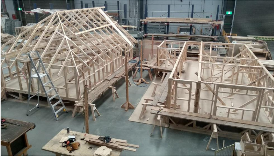
Figure 11. Victoria University Polytechnic Sunshine campus. The trades floor of the building trades with partially completed timber framed structure built on half-height walls for safety of the students.
