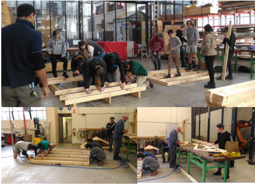
Figure 6. Shed construction. Initial stage construction where groups were each responsible for a separate component.
