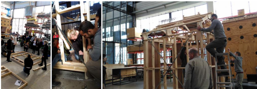
Figure 7. Shed construction. Assembly of components together where groups now have to negotiate theirs with other groups' components.
