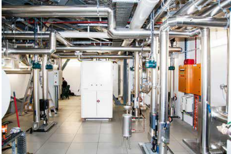
Figure 6.2: The plant room with the Organic Rankine Cycle (ORC) in Building 11 University of Technology Sydney. UTS Building 11.
