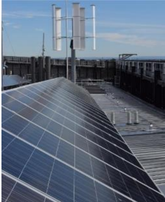
Figure 6.4: The PV panels and the wind turbine on the rooftop of Building 11, University of Technology Sydney. UTS Building 11.
