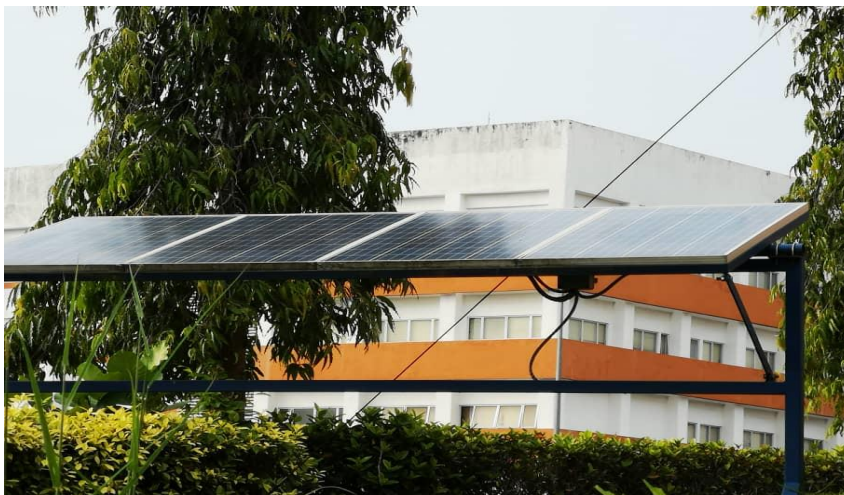
Figure 5.153: Plate-PV for solar energy collector. UniKL MFI field research area.
