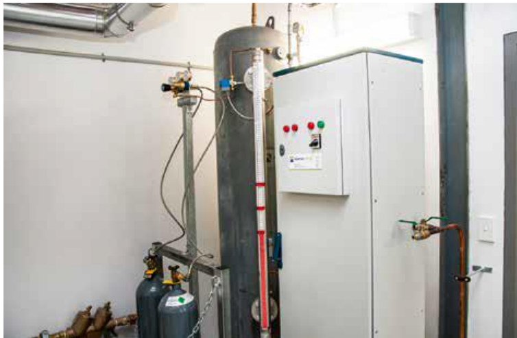
Figure 6.3: The fluid thermal expansion system in Building 11 University of Technology Sydney. UTS Building 11.
