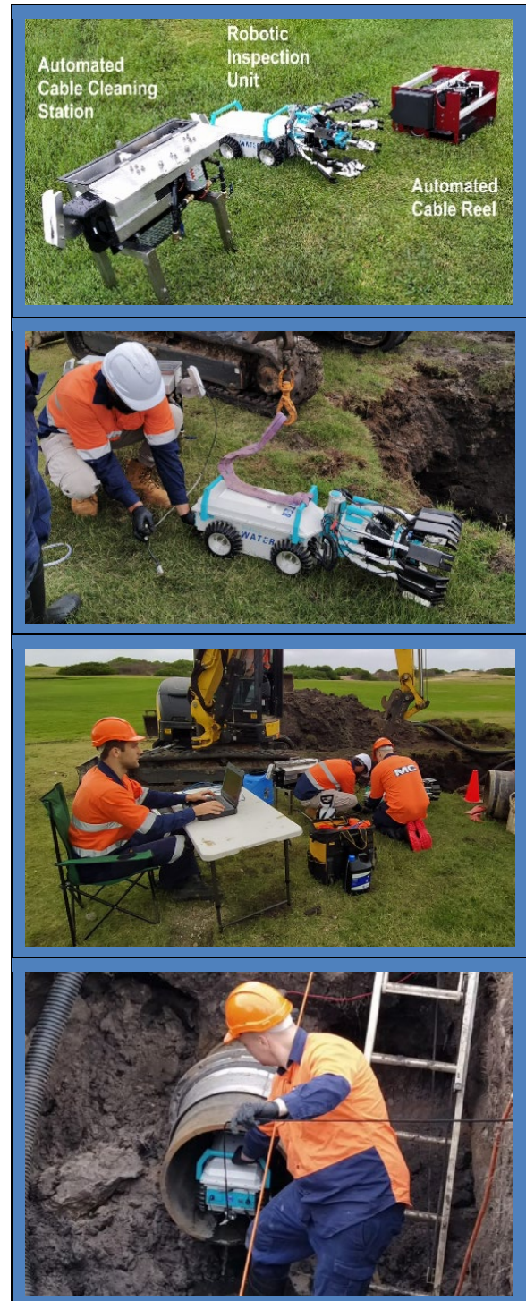
Figure 3 Field deployment during Feb 2021 in a Rising Main at Sydney Water
