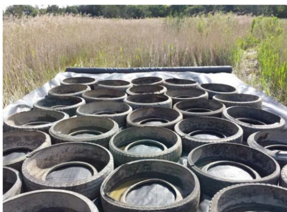
Fig. 8 Tyre cells ready to be filled with the granular infill material in a field project
