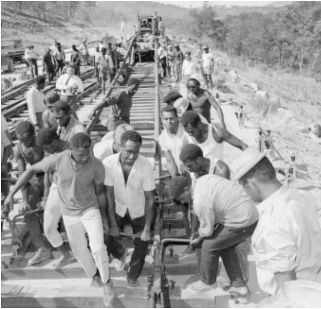
Fig 2. Islander track-layers positioning the 360 foot rail over sleepers on the standard-gauge railway line, Upper Swan, Western Australia, February 1965.
