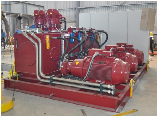
(c) Hydraulic power unit
