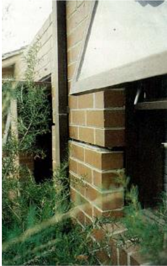
Figure 1.1 A damaged building in Melbourne caused by shrinkage settlement of foundation over-drying expansive soil after Considine (1984)
