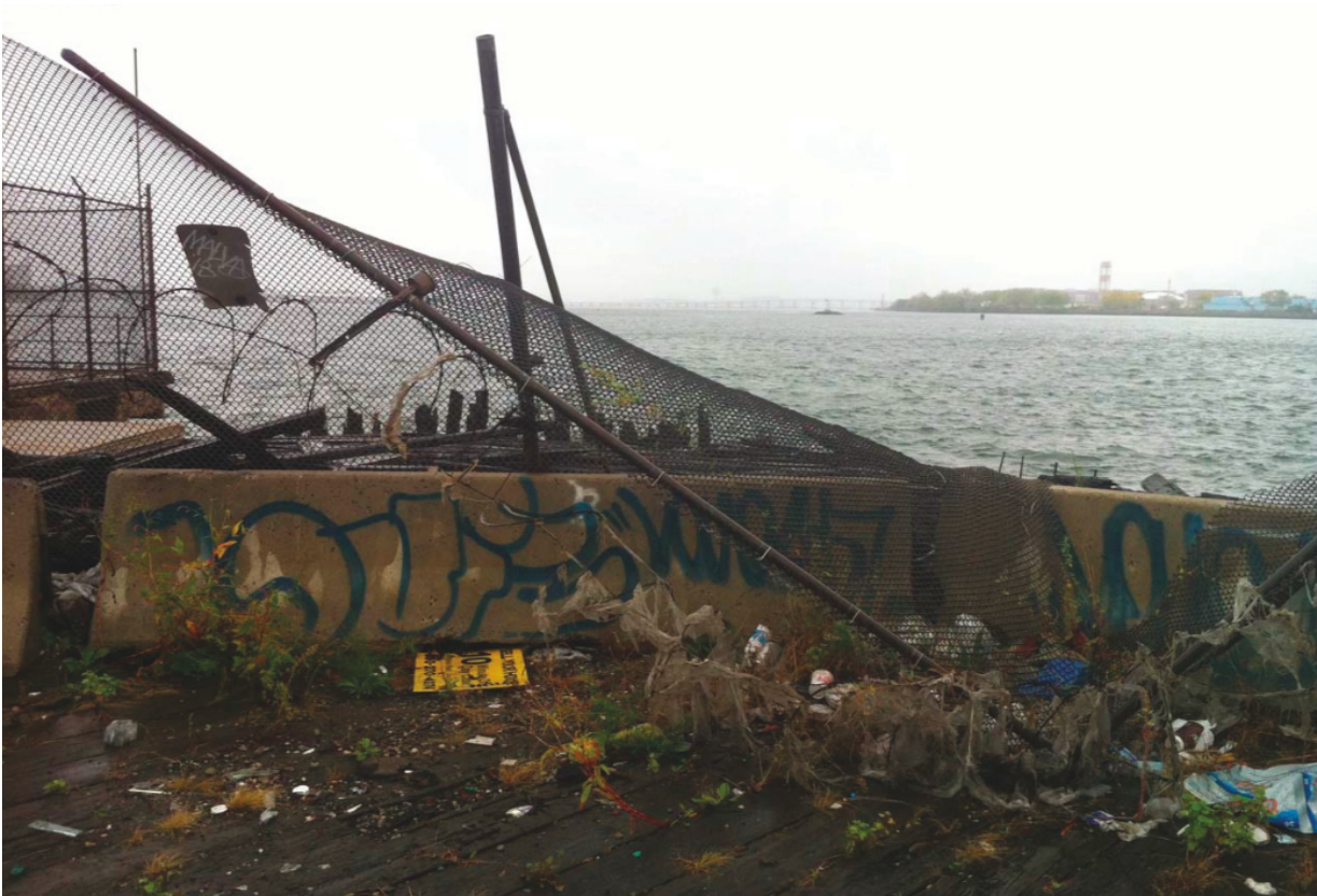
Figure 6 The street end pier on East 132nd Street in Port Morris has not been repaired after an explosion in 1989
