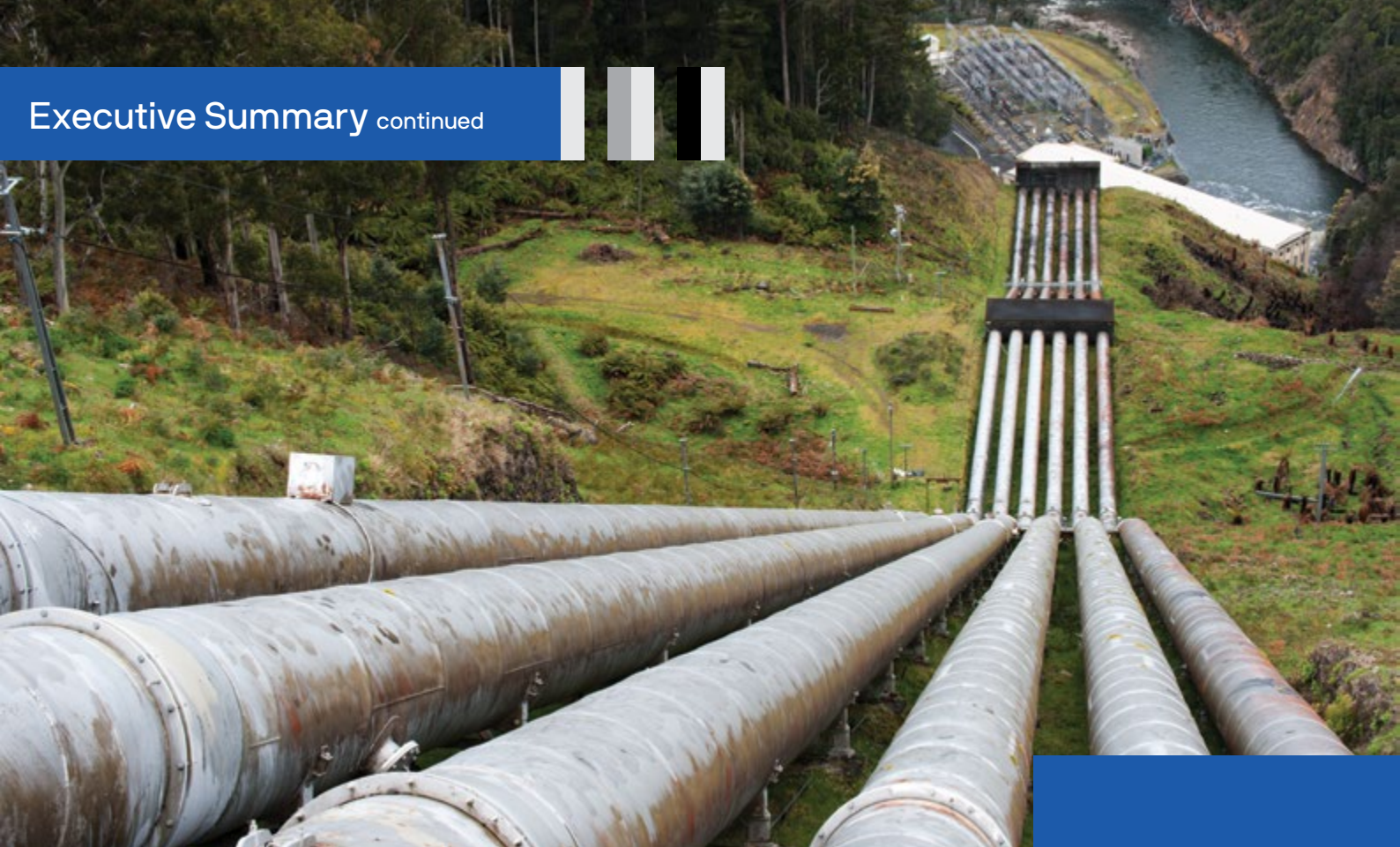
Penstocks feeding the Tarraleah Power Station, a pumped-storage hydroelectric power station in Tasmania, Australia.
