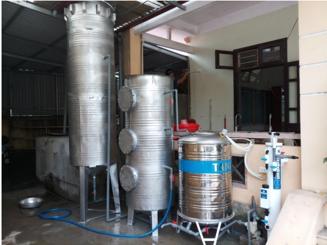
Figure 6.1. Digital picture of real water treatment system at the Hoang Tay children care centre, located at Ha Nam province in Vietnam
