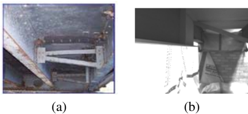
Fig. 5. a) A real bridge structure environment; b) Experiment setup
